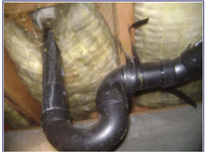
Leakage from the drain line below the shower enclosure in the lower level bathroom
