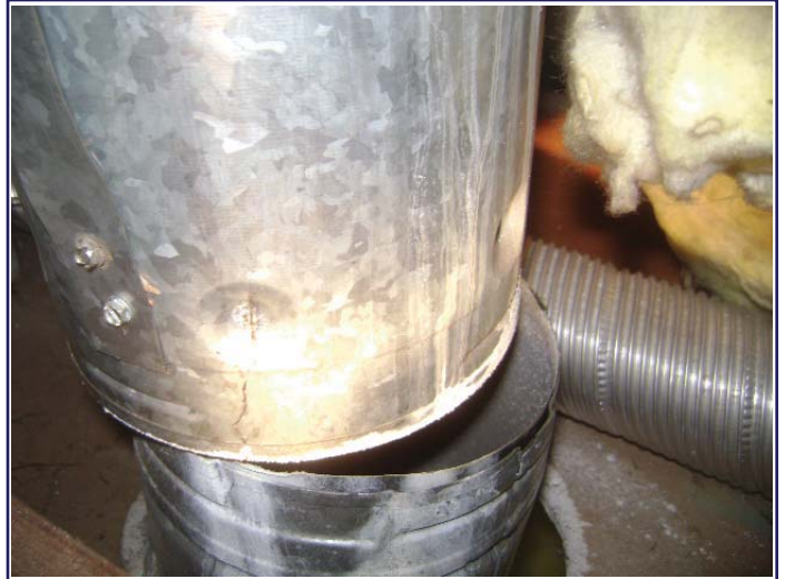
Furnace's flue pipe is disconnected in the attic
