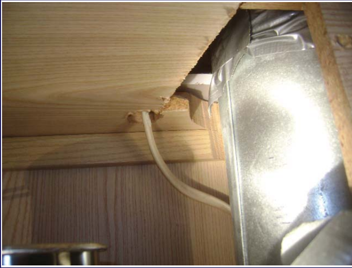
Unprotected electrical wiring in the kitchen cabinet above the stove
