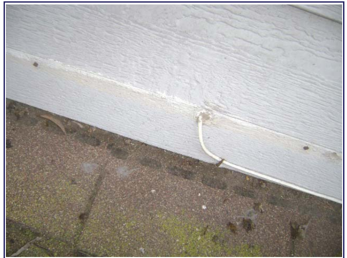
Exposed roof nails above the rear of the house
