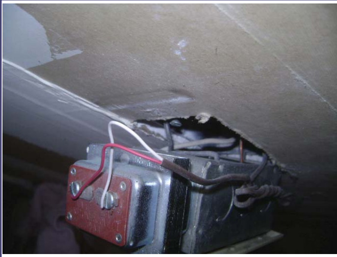
Exposed electrical wiring ( loose box ) in the garage at the firewall
