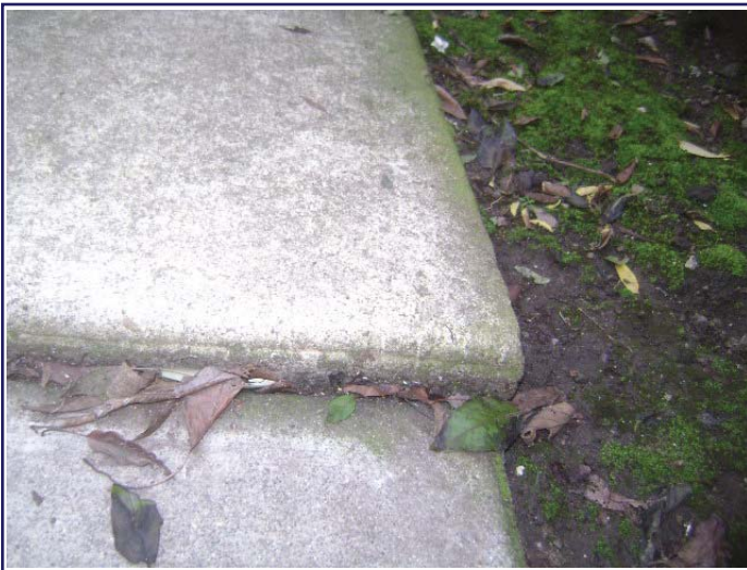
Heaving to a section of the concrete walk, located on the right rear side of the house
