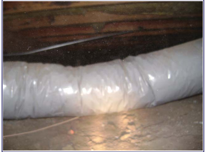
Heat duct in the sub area in contact with the soil
