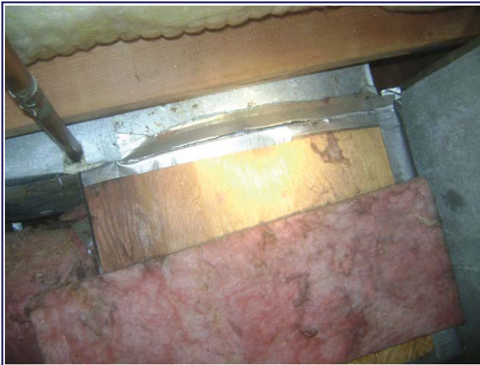
Plywood covering the side of the sheetmetal plenum in the sub area
